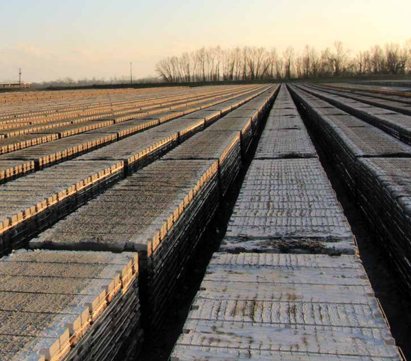
LEFT Concrete mattresses made at the St. Francisville Casting Fields are sunk into the Mississippi River to create revetments that fix the river's banks and maintain navigation channels.
